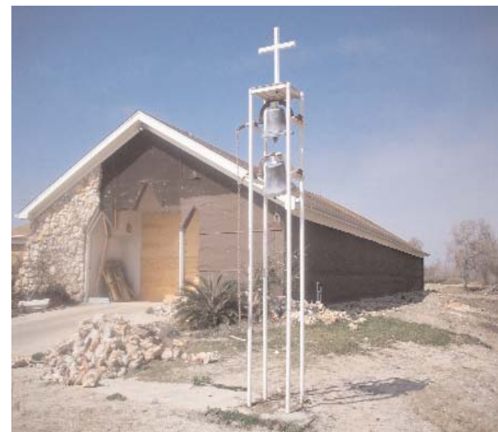
Bay Vue UMC suffered extensive damage during Hurricane Ike.
